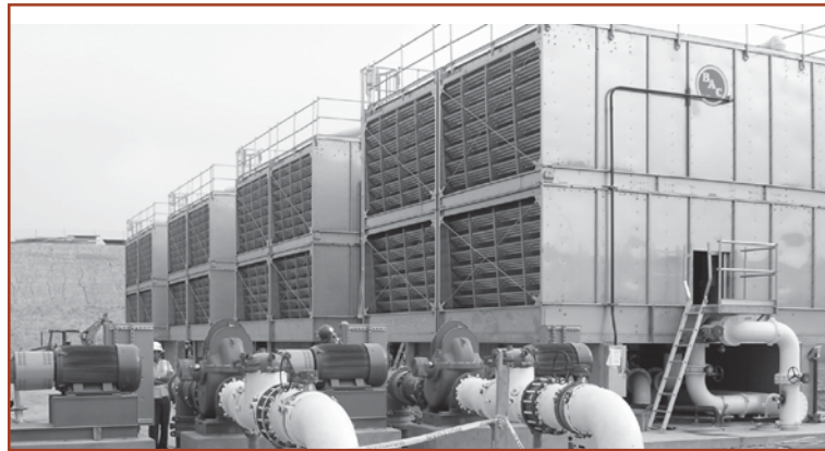
Fig. 1 Cooling tower pumps
